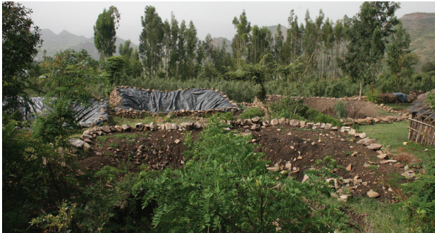
Here a farmer has multiple water harvesters. The nearest is still under construction.
